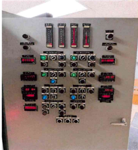
Figure 6 Smith WTF Analog Controls (Installed 1995)
