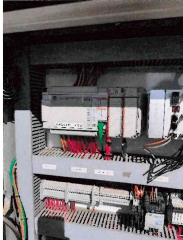
Figure 10 Fleetwood Lift Station Obsolete Micrologix PLC System
