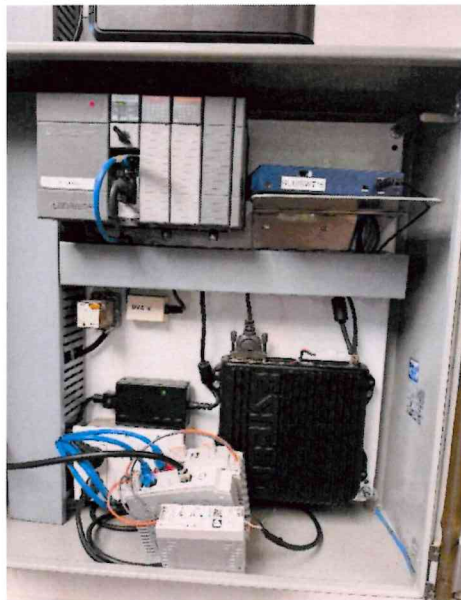
Figure 7 Main Office obsolete Central PLC System
