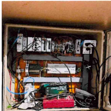
Figure 12 Reservoir Obsolete Micrologix PLC System
