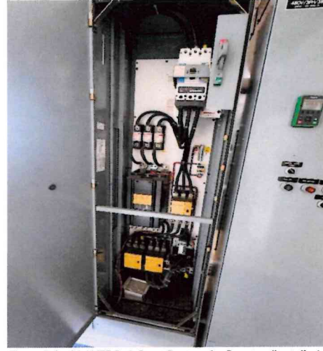
Figure 7 Smith WTF Soft Start System for Booster (Installed 1995)
