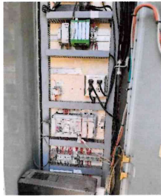
Figure 16 Well 8 Obsolete Micrologix PLC System
