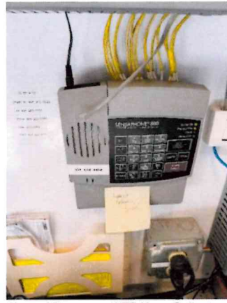
Figure 4 Thompson WTF Alarm Callout System
