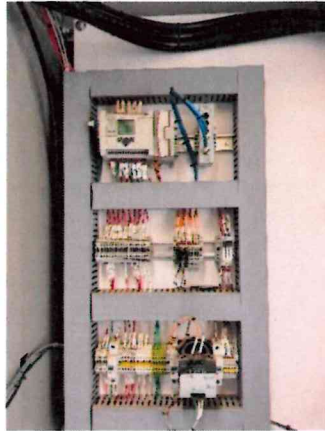
Figure 13 Well 1A Obsolete Micrologix PLC System
