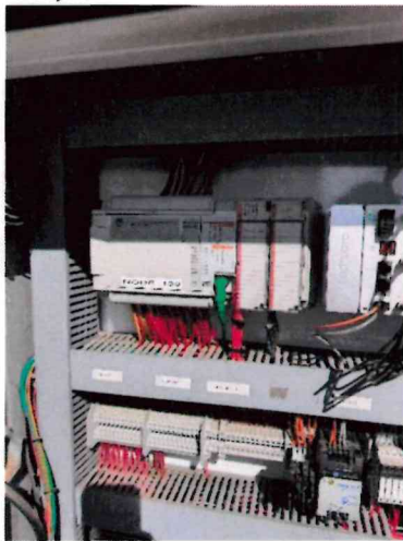
Figure 10 Fleetwood Lift Station Obsolete Micrologix PLC System
