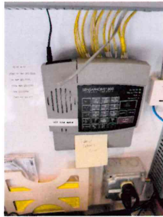
Figure 4 Thompson WTF Alarm Callout System
