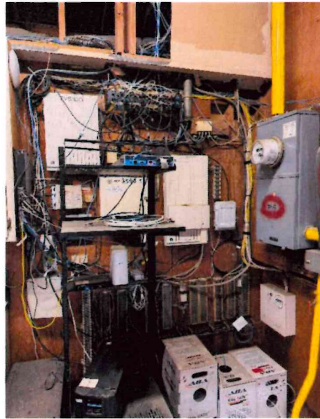
Figure 8 Main Office obsolete Comm Room, No Documentation or labeling
